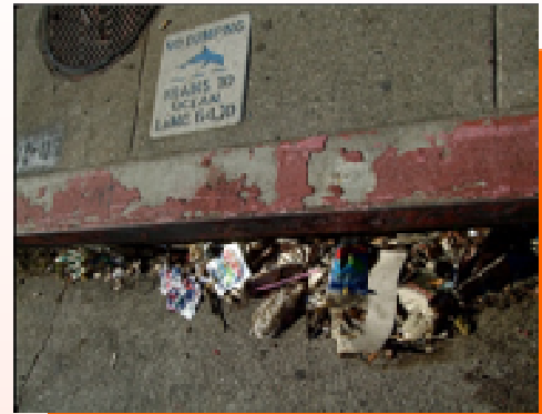
Figure 2 – Trash accumulating next to catch basin
